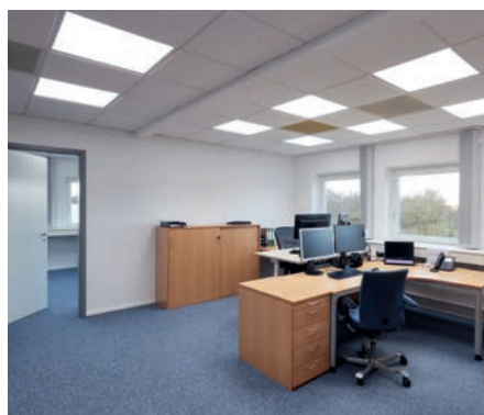
Modern VIVARES Zigbee light management system – installed in the old office building.
